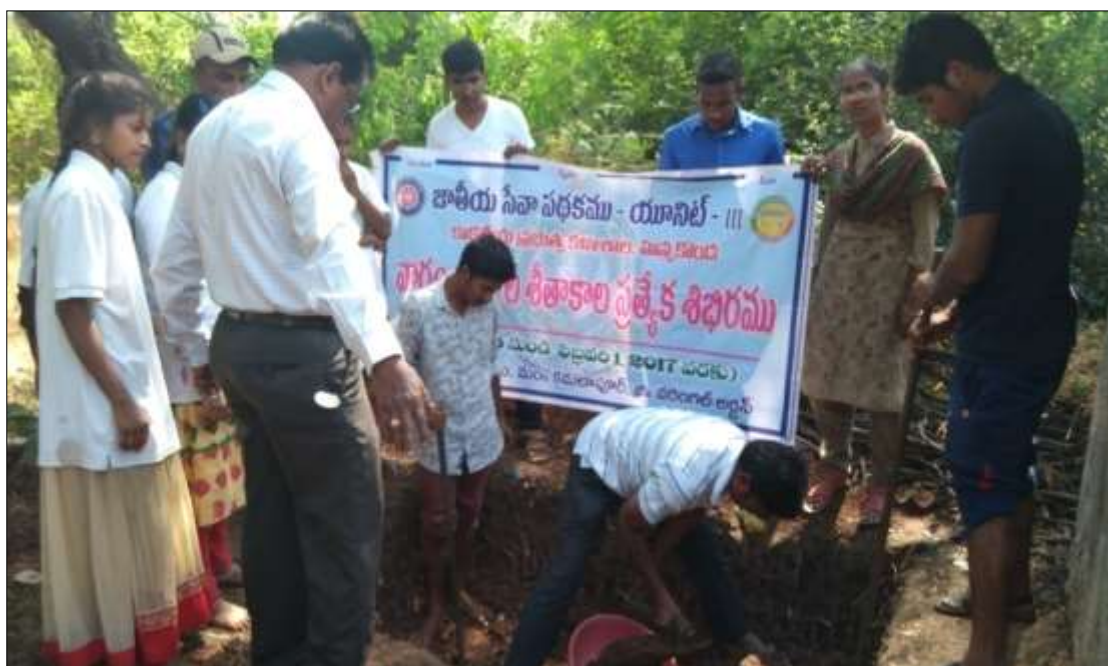
The NSS III Unit (commerce) participating in construction of Water Harvesting Pits on 30-01-2017 at Marripally Gudem Village
